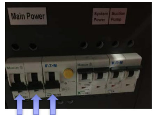
Figure 5-3: Main Power Breakers
